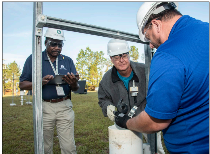
SRS Engineers Inspect a Solar-powered MicroBlower™.
