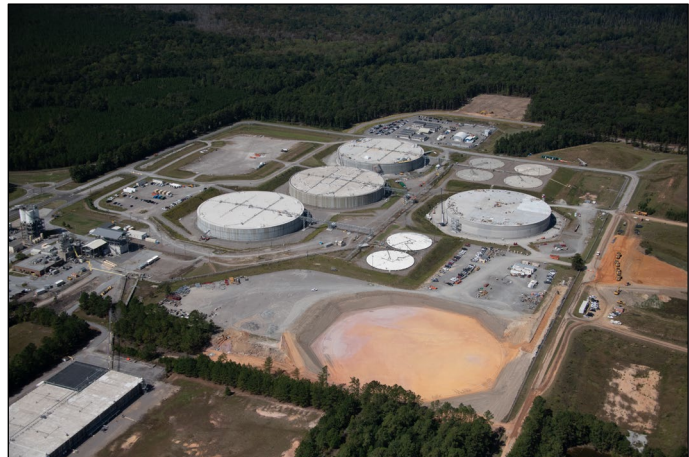
Excavation and Groundwork were Initiated for SDU-11 and SDU-12, the Final Mega-Vaults Planned for Construction.
