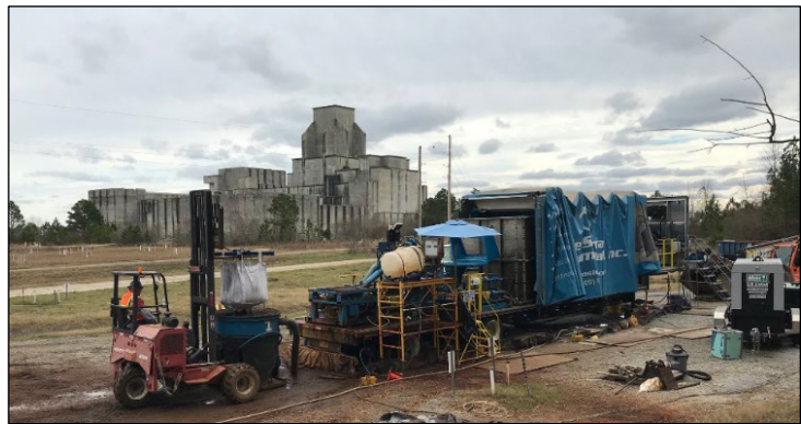
A Subcontractor Loads Zero-Valent Iron Filings during Injections to Support Installation of the P-Area Reactive Barrier
